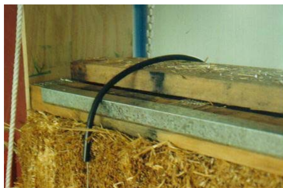
Figure 3: View of top plate assembly showing sleeved wire loop. (Photograph P. Florence)
